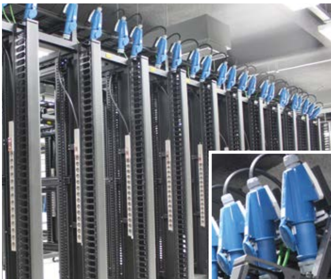
Internet Data Center, South Korea
