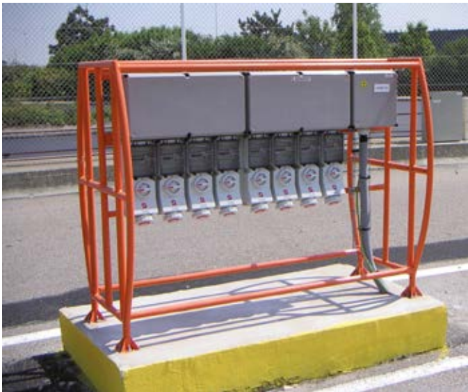
Container Terminal, Le Havre, France
