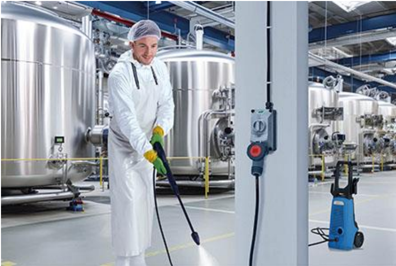
Photo 1 (MENNEKES): The wall mounted receptacle DUOi in the food processing industry.
